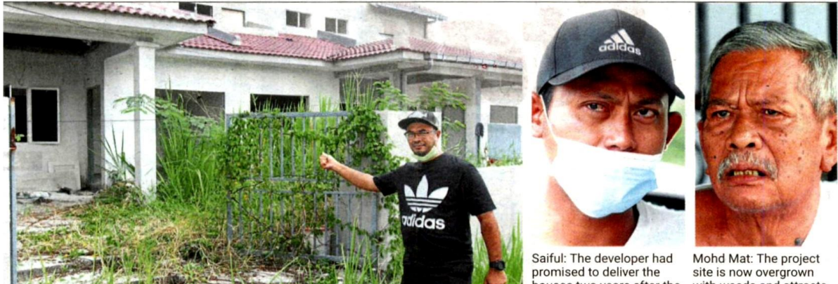
Wan Zalmi in front of his unfinished unit at Block A of Kampung Delek. Work stalled after 75% of the house had been completed. — KK SHAM/The Star
